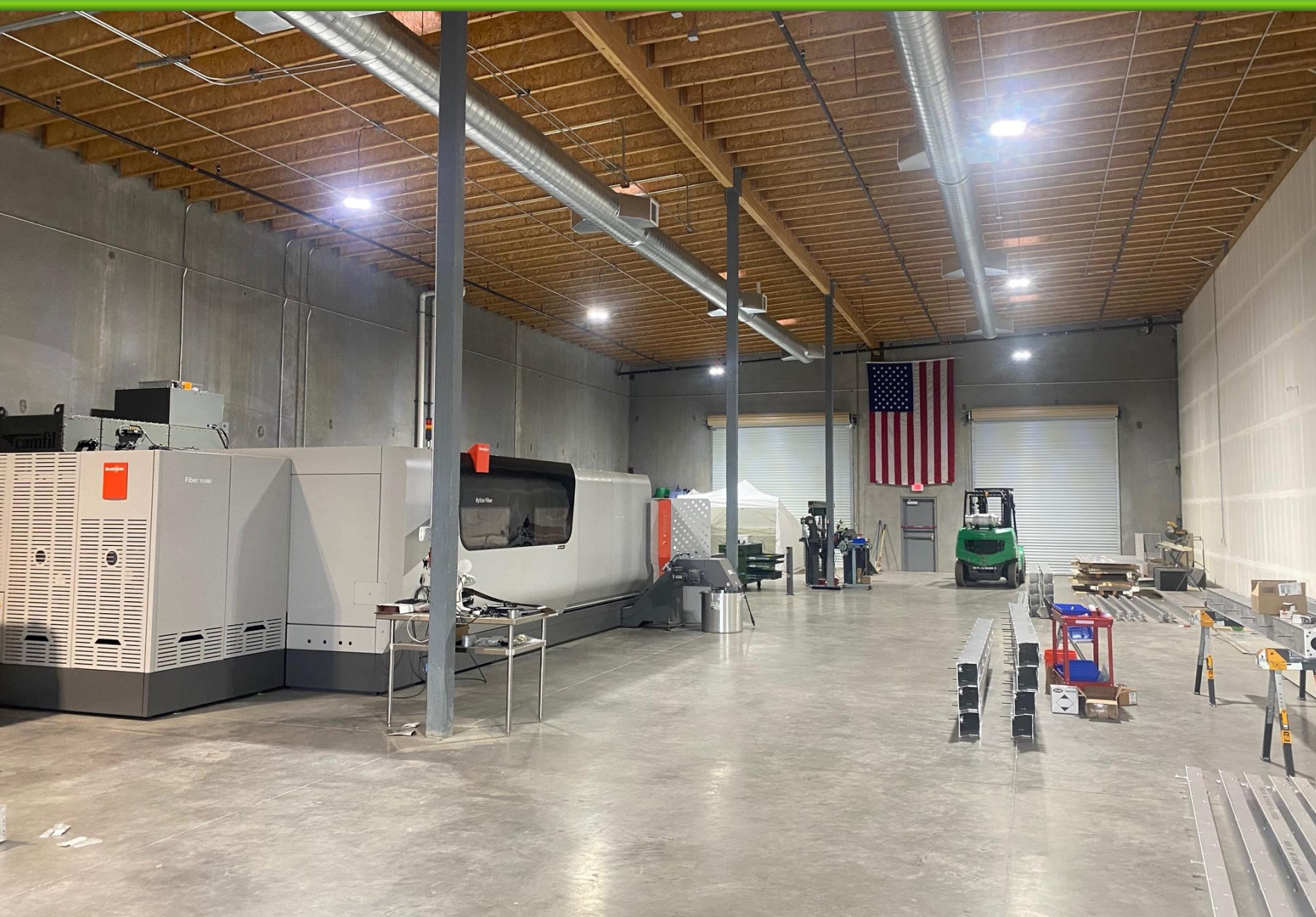
Bystronic Laser for precise cutting and part production at the ARES Manufacturing facility (Las Vegas, NV)
